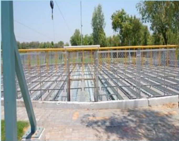
Biogas Generation in ETP
