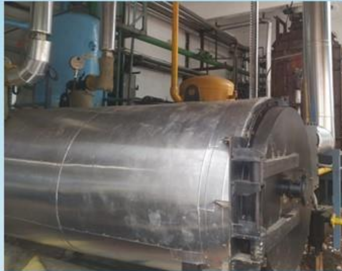
Hot Water Generator
