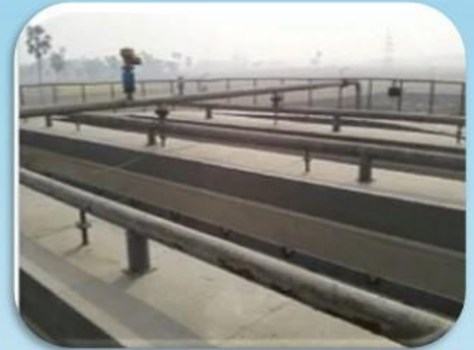
Biogas Generation at ETP
