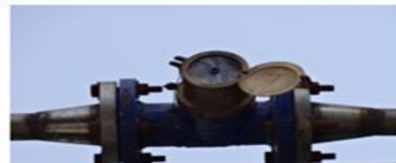
Water Flow Meter
