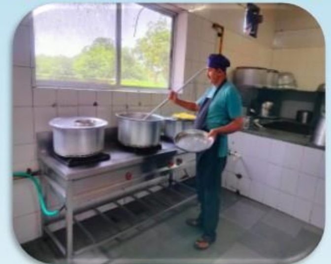
Biogas Generation utilization at Canteen
