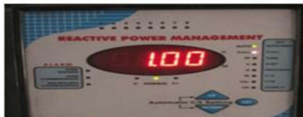
Power Factor Meter
